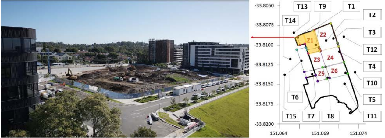
Figure 2. Construction site in Zone 1 (left) and the locations of 15 sensor nodes for emission monitoring in Melrose Park and residential areas (right) [20, 3]
